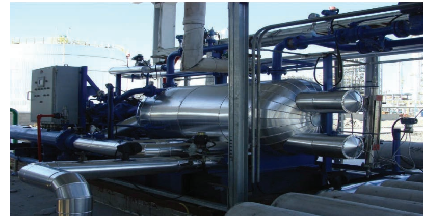
Flare Gas Recovery
