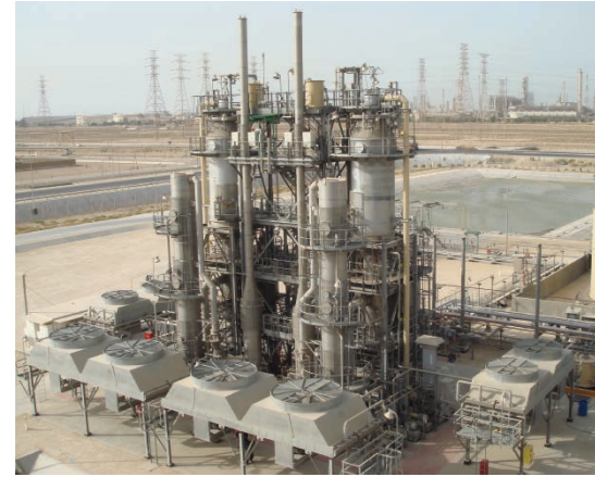
Thermal Oxidizer System
