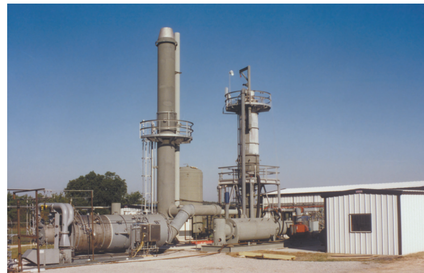
Three stage combustion system at Honeywell UOP Callidus research facility
