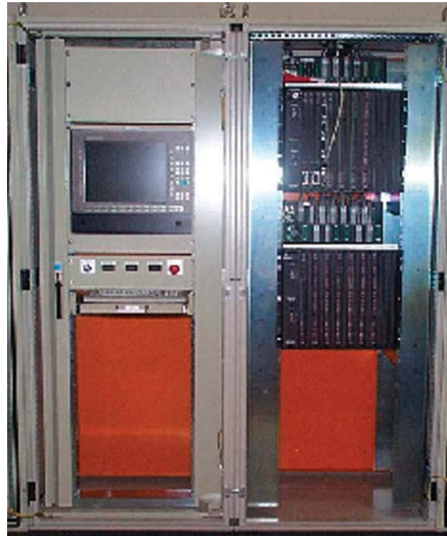
Figure 1 ■ Typical UOP LHCS Retrofit Cabinet Layout
