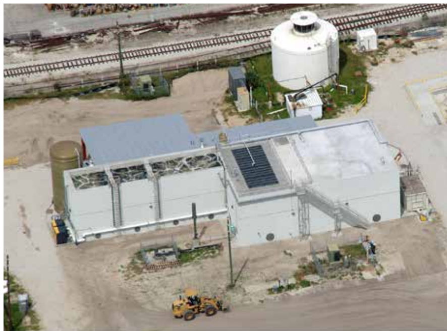
As the beverage manufacturer's wastewater flows through the treatment system, it goes through (from left) the equalization tank, upflow anaerobic sludge blanket reactor (UASB), and immobilized cell bioreactor. Honeywell UOP
