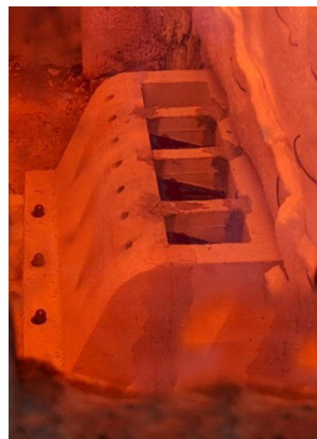
CUBP Steam Cracker Burner Firing 100% Hydrogen
