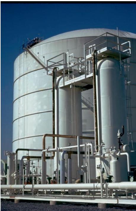
Multiple bed adsorption for H 2 O and CO 2 removal from natural gas before methane liquification.
